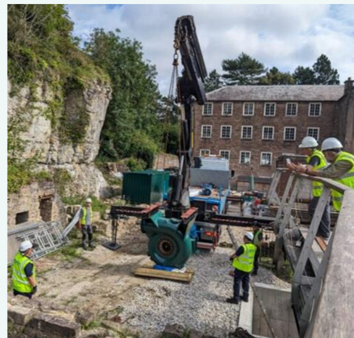
Image: The operational watermill at Cromford Mills ( far left ) and its construction ( left ). © Cromford Mills / The Arkwright Society.
